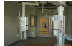
Medical gas booms and lights in burn ICU
